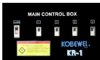
Main Control Box
