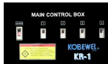
Main Control Box
