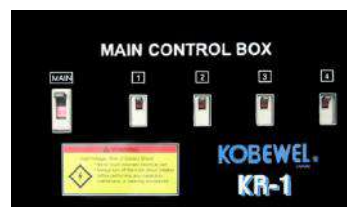
Main Control Box
